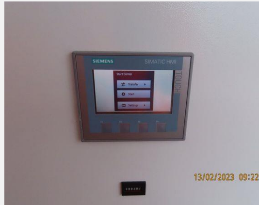
Bedienings- en besturingsinstallatie - Supervisory Control and Data Acquisition (SCADA-systeem) ( 1 )
