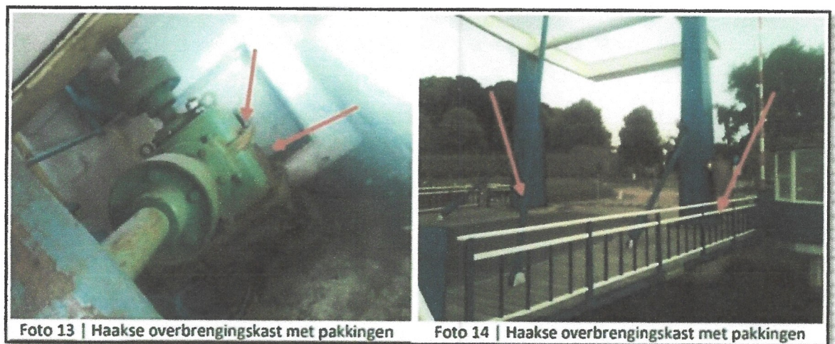
Figuur 4: Asbest in pakking.
